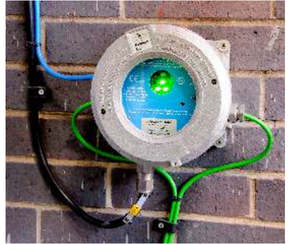
5. The Earth-Rite RTR in a permissive condition.
